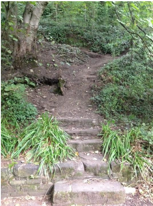
Decayed Steps in 2016
